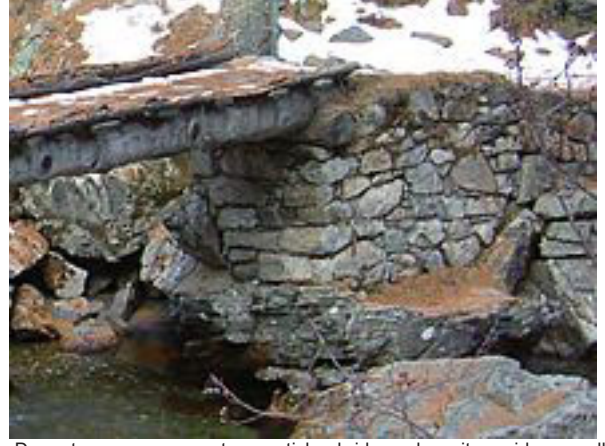
Dry set masonry supports a rustic log bridge, where it provides a well - drained support for the log (which will increase its service life)
